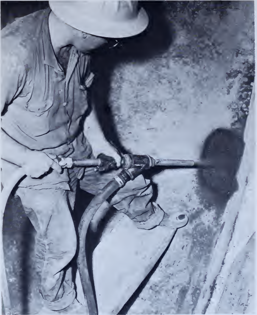
Figure 181. —Application of replacement mortar. The mortar should be applied on dry contact surfaces that are as clean as a freshly broken piece of concrete. PX-D-33057.
